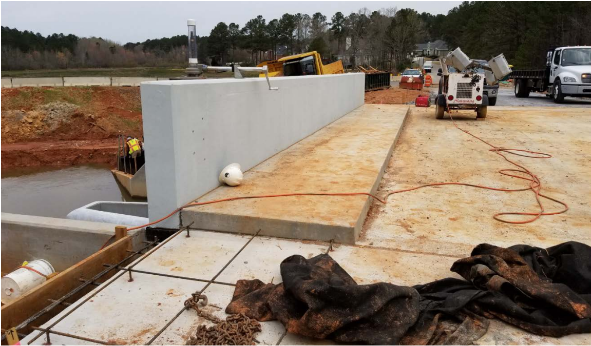
Photo 1: Bridge construction continues over the spillway. Utility work is also in progress. (03/23/2018)
