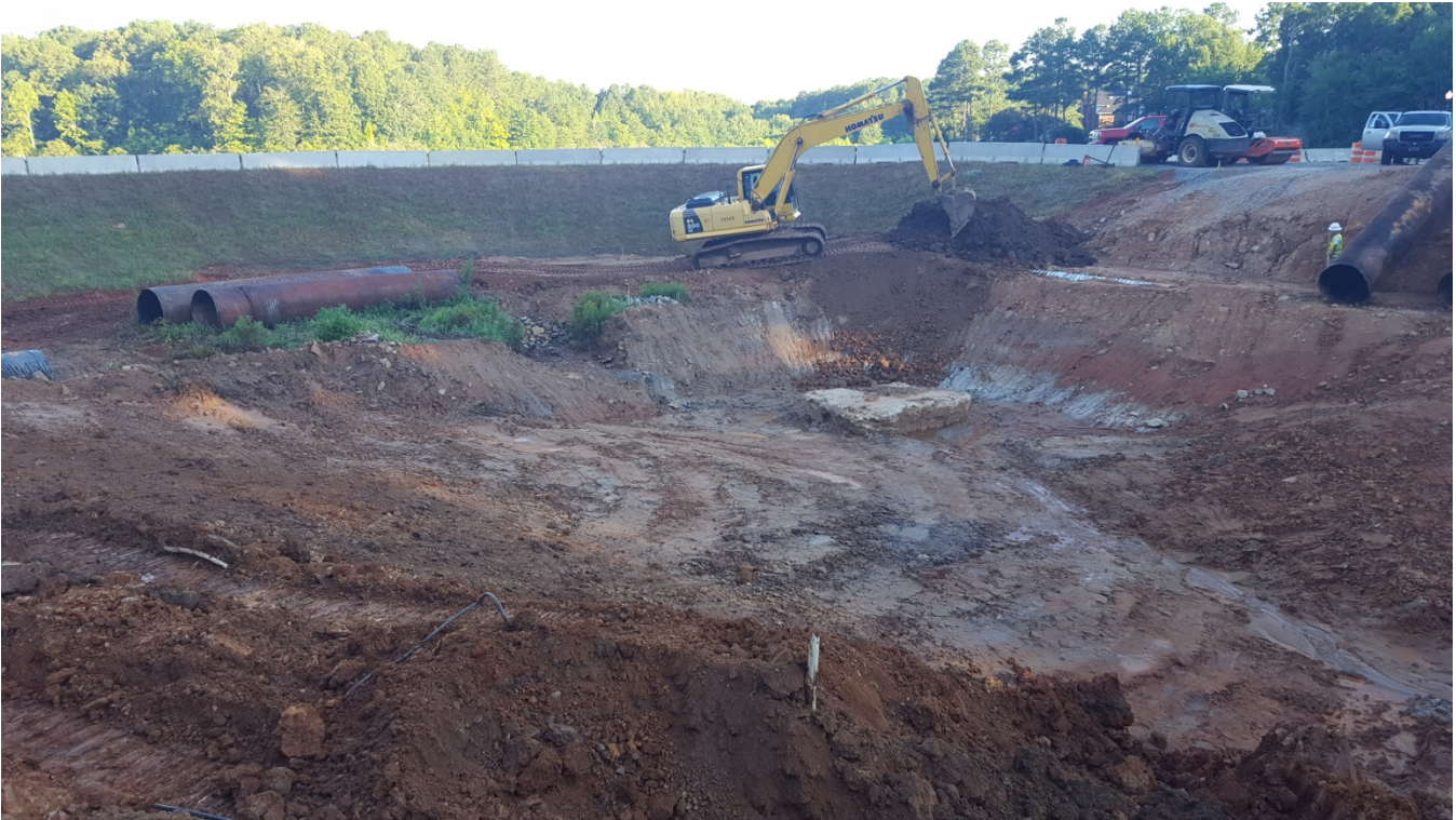
Photo 1: Emerald Lake Dam after the demolition and removal of former spillway and outlet control structure. The temporary cofferdam and road detour is visible in the background.
