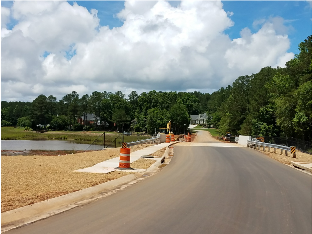
Photo 1: Photo is of new dam, bridge and road. Remaining work activities include construction of retaining wall (see left side of road on far side of bridge), shoulder stabilization, and refilling of the lake.
