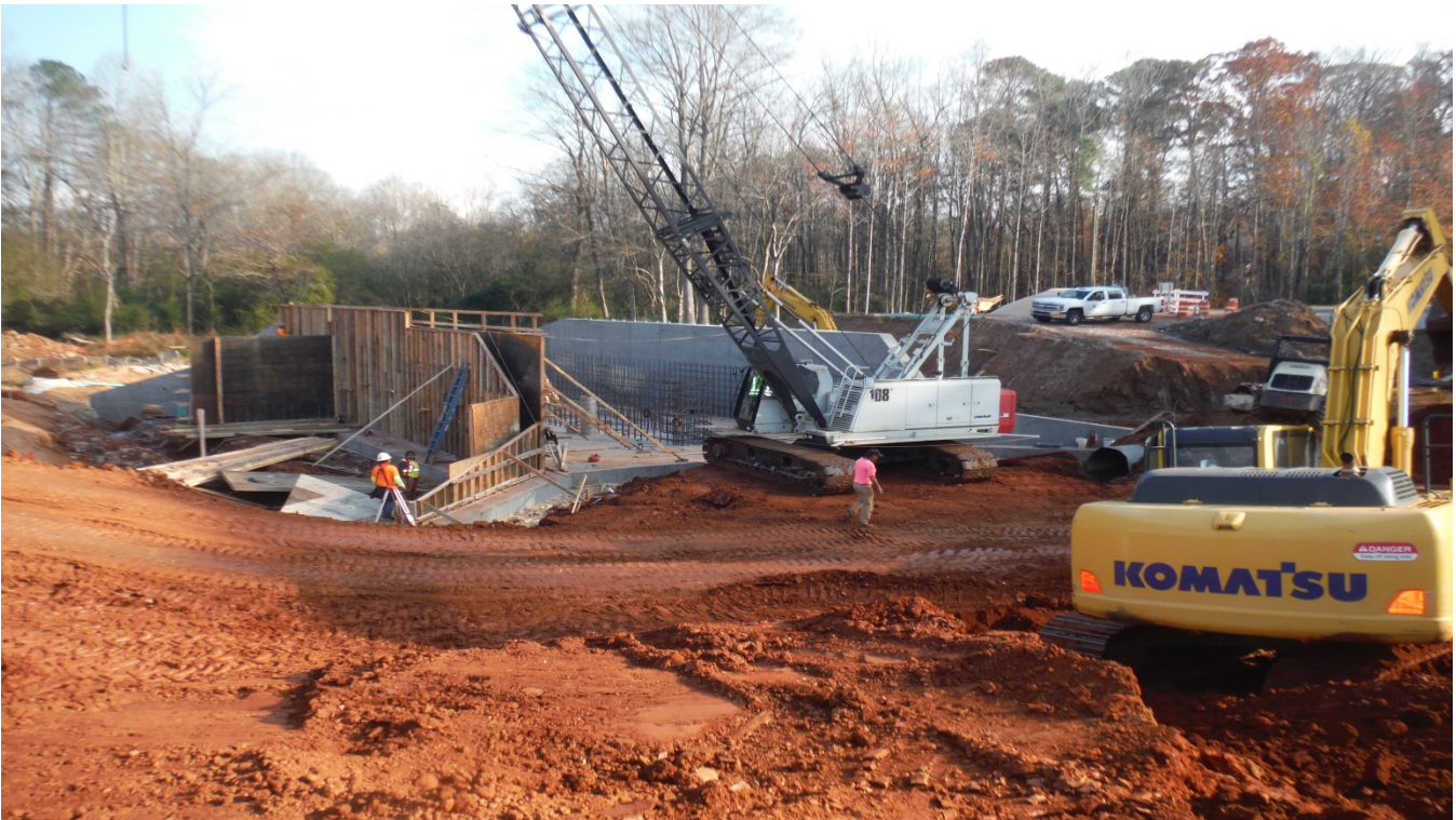
Photo 1: Forming of one wall for concrete pouring. Second wall has been poured. (12/1/17)
