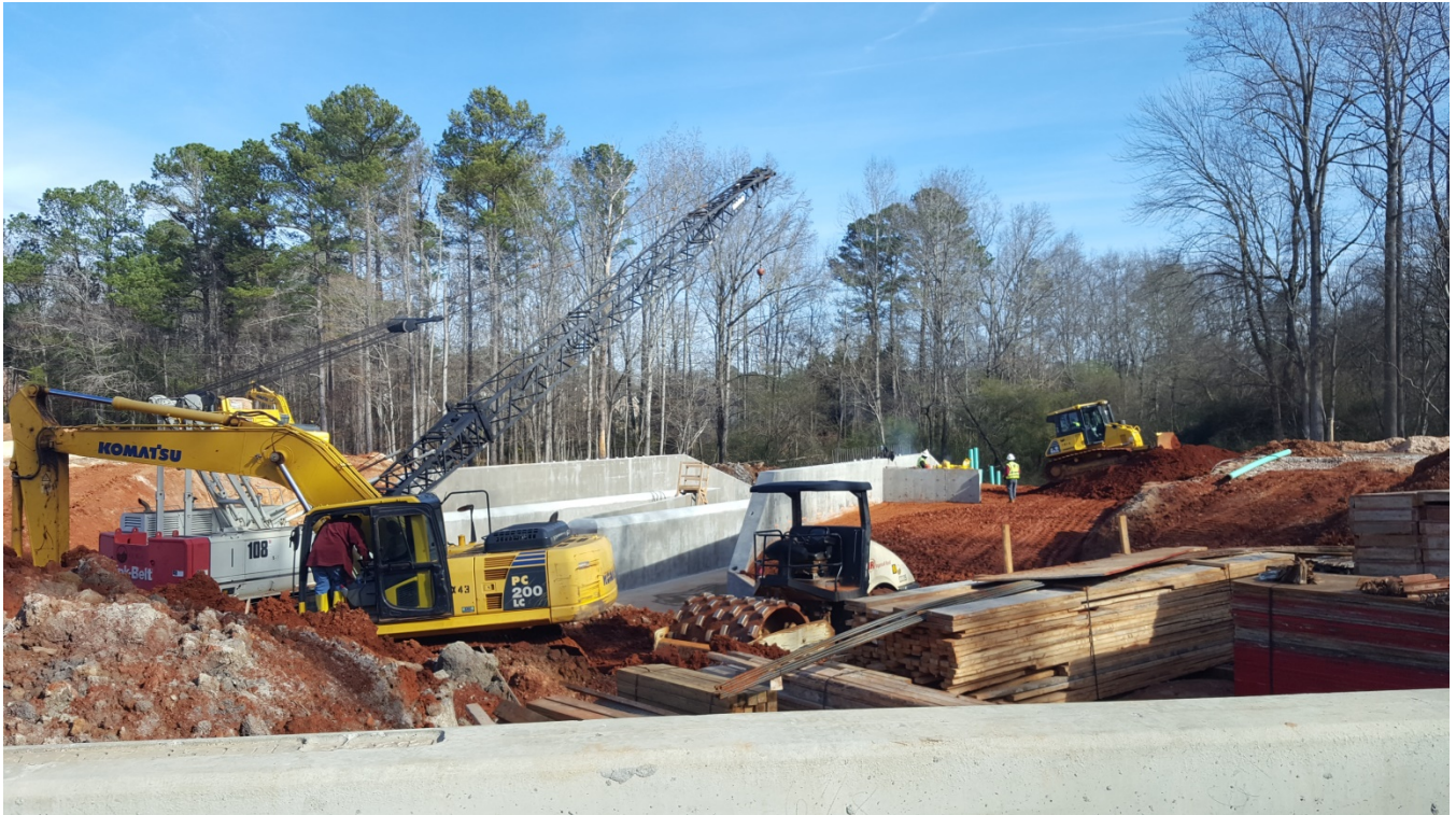
Photo 1: View of Emerald Lake Dam spillway. Backfill operations underway after wall construction. (12/26/17)
